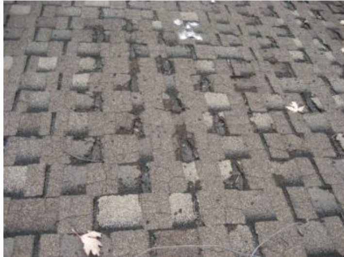
Composition shingle condition
