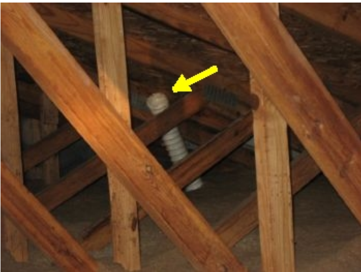
Bath fan vented to attic space
