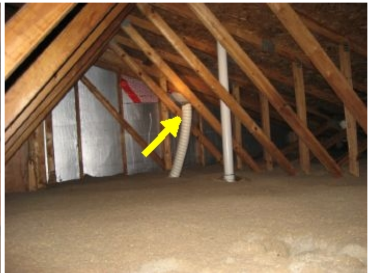
Master Bath fan vented to attic
