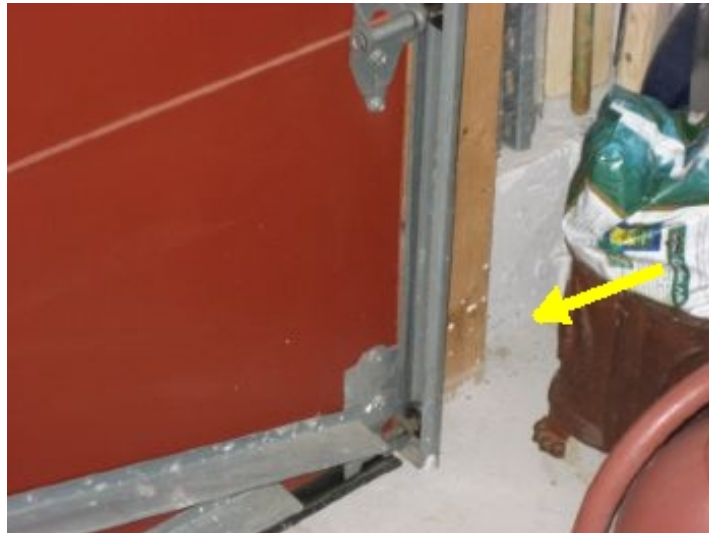
No Door Safety Reversing System Installed
