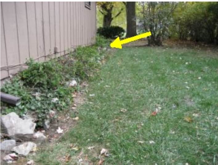
Reverse Grade at rear of home
