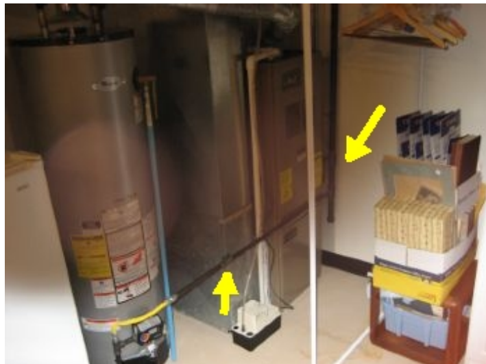
Water Heater/Furnace Gas Shut-offs
