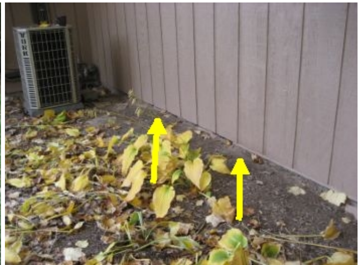
Insufficient Grade separation at Siding
